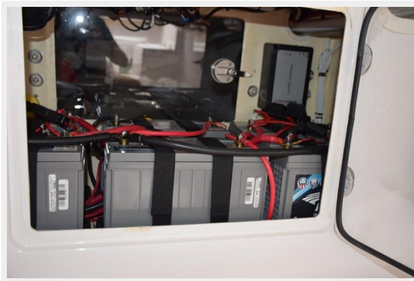
Northstar batteries in sealed hatch under console
