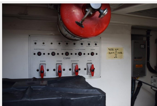
Battery switches and ER fire system
