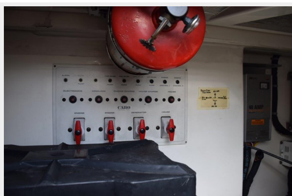
Battery switches and ER fire system
