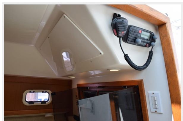
VHF radio inside cabin, electrical panel
