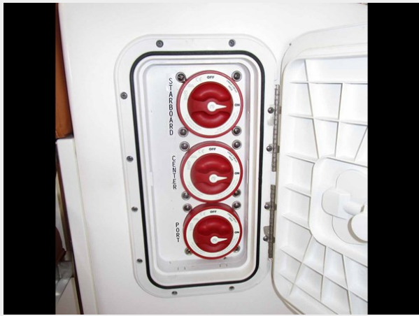
Engine Battery Switches
