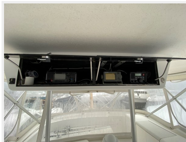
Overhead electronics box
