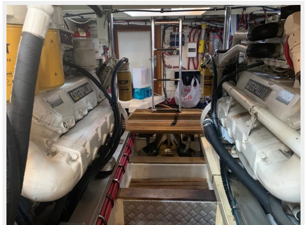
Engine Room Looking Forward
