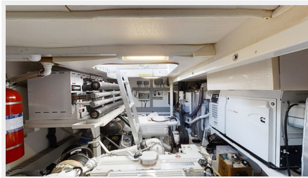
RELENTLESS 2018 Prestige 560 Flybridge Motoryacht: Engine Room
