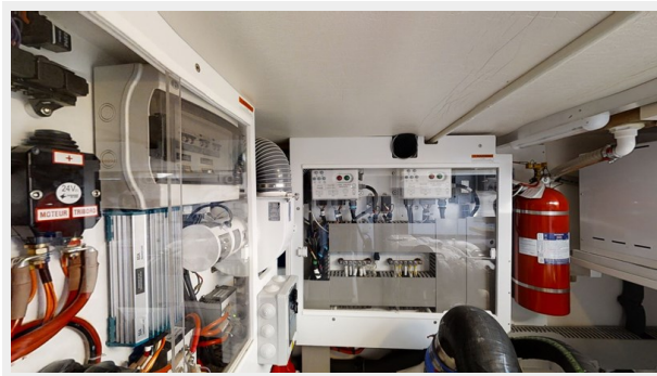
RELENTLESS 2018 Prestige 560 Flybridge Motoryacht: Engine Room
