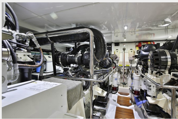
Engine Room Starboard
