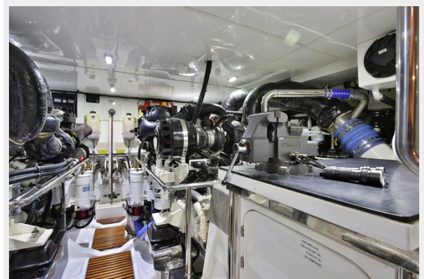
Engine Room Portside
