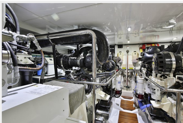
Engine Room Starboard
