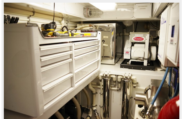
Pump Room - Tool Box - Compressor
