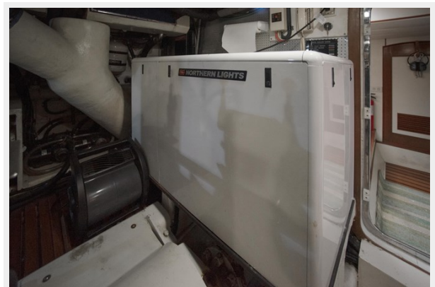
Generator Stbd Side
