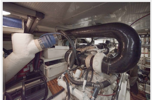
Engine Room Port Side
