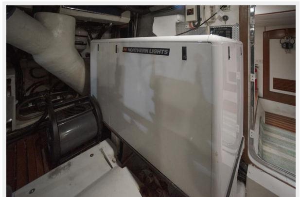
Generator Stbd Side
