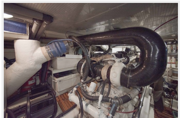
Engine Room Port Side
