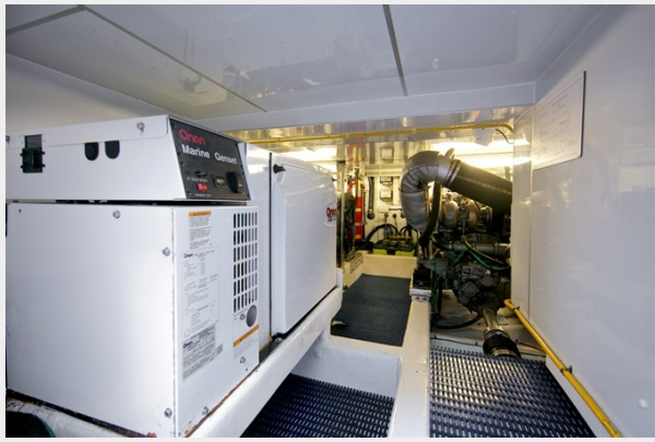
Genset looking forward into engine room
