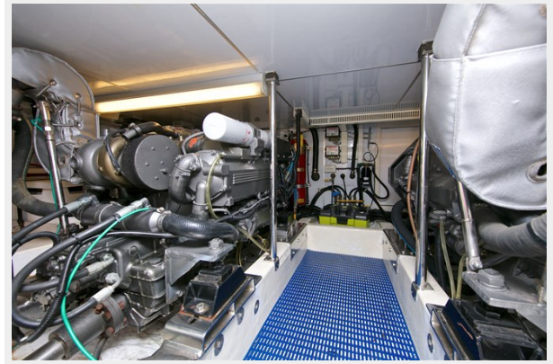
Well maintained engine room
