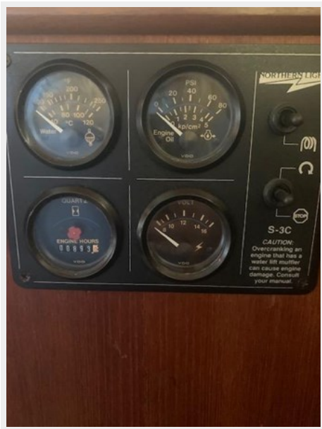
1984 Sundowner Tug 30 generator panel
