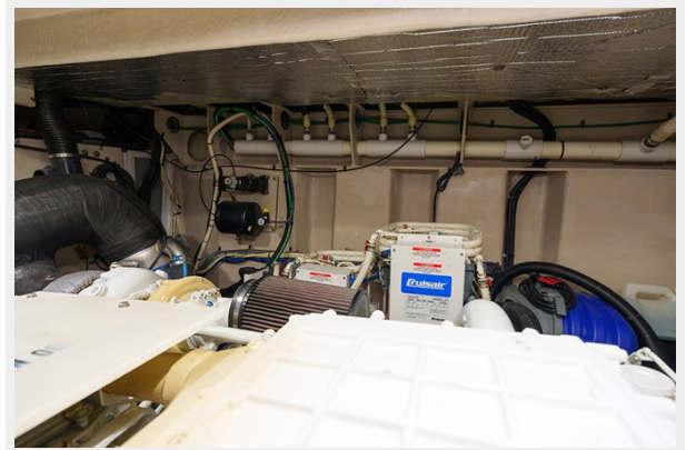
Engine room view 4
