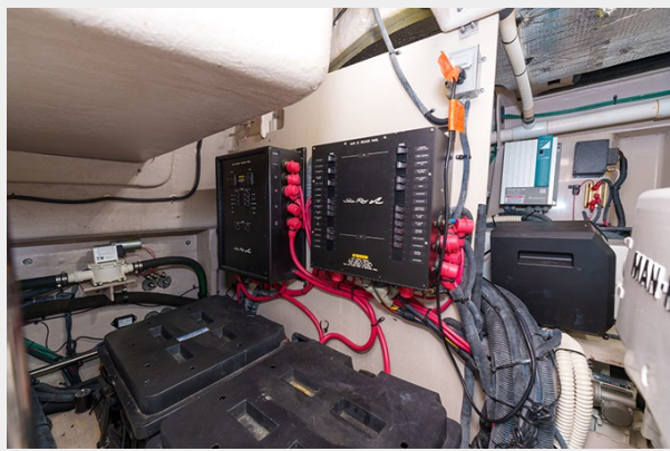
Engine room view 3
