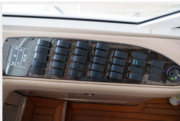
Switch control panel at the helm
