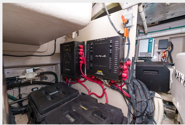
Engine room view 3
