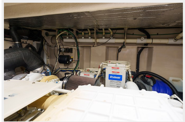
Engine room view 4
