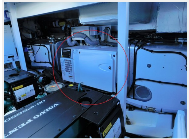
14-Cummins Onan Generator
