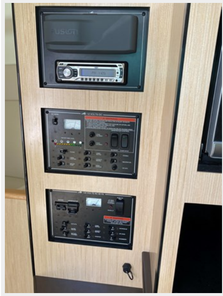
19-AC DC Control Panel
