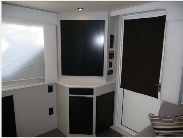
Main Salon and Electrical Panel
