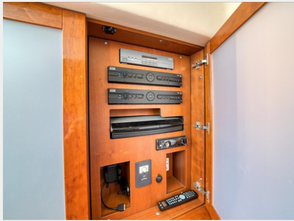
Salon Control Panel 1
