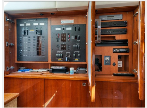
Salon Control Panel 2
