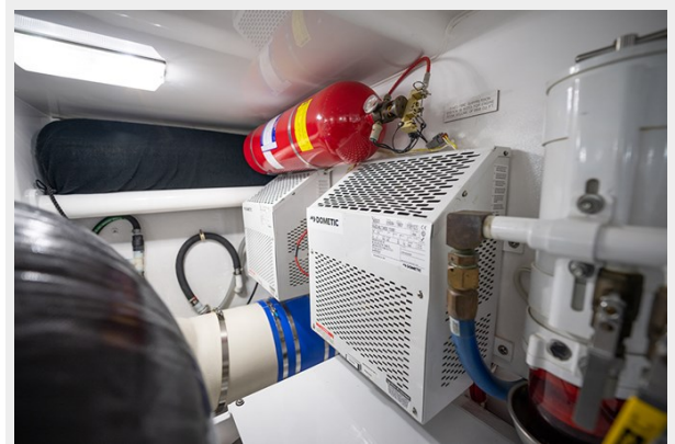
Fixed fire suppression system
