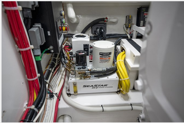
Engine room view 5
