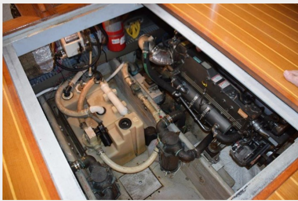
Hatch open above engine room
