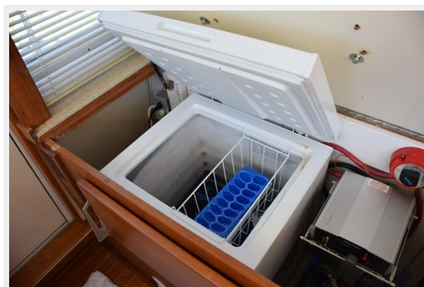
Freezer under helm bench
