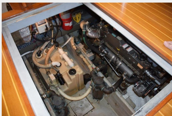
Hatch open above engine room
