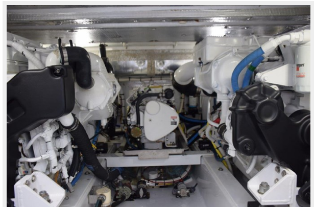
Engine Room with generator centerline
