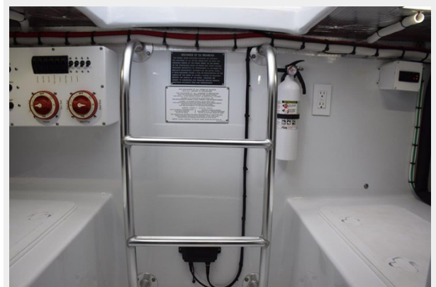
Forward pump room area
