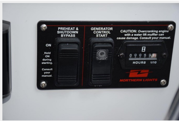
Northern Lights generator panel, under 70 hours
