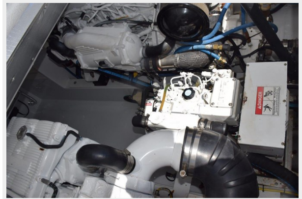
Generator view from above
