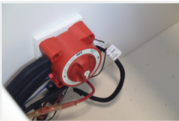
16. Dual Battery Switch
