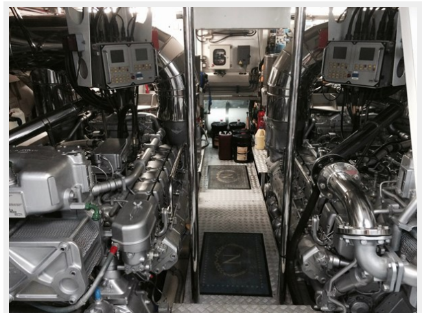
Mangusta 107 - Engine room
