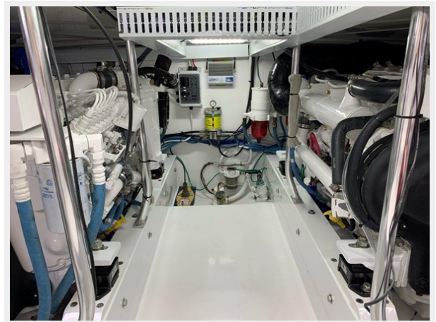
Strengthened engine mounting beds
