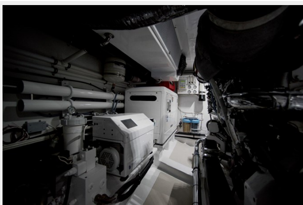
Generator and Watermaker
