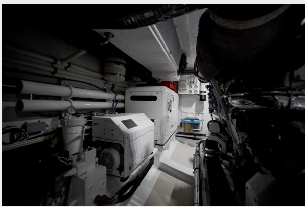
Generator and Watermaker
