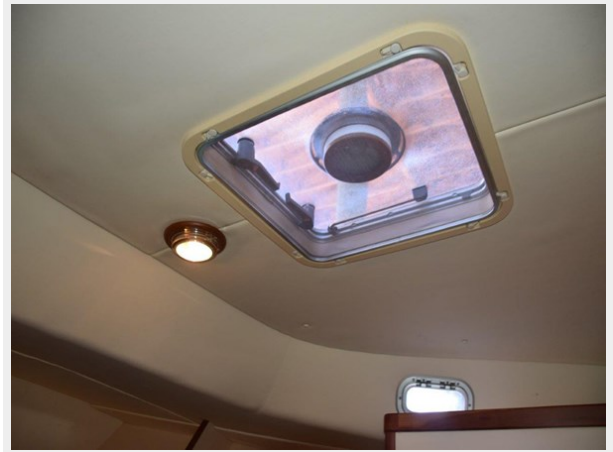
Overhead hatch with solar vent fan
