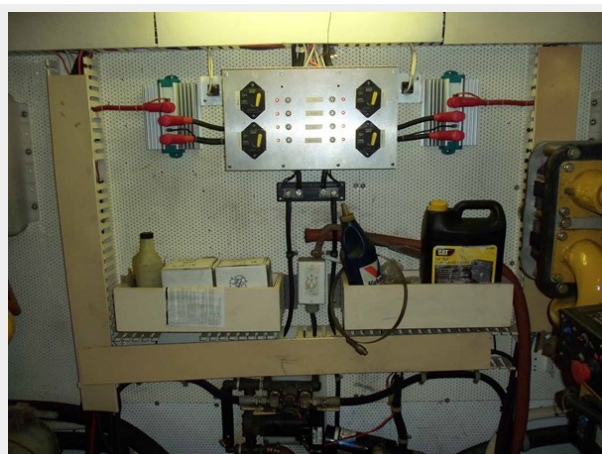
Engine Room Forward
