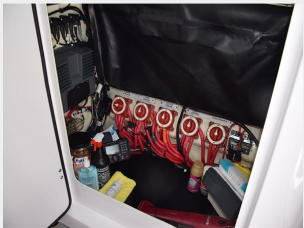
Battery switches and access to console equipment
