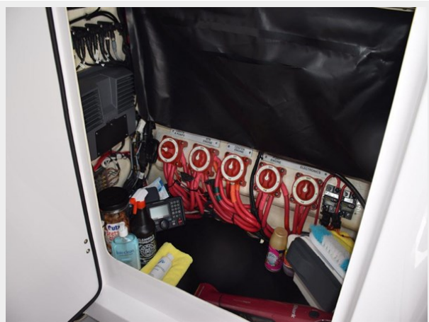
Battery switches and access to console equipment
