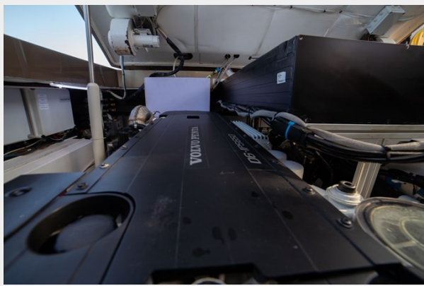
Hydraulic Lift Engine Compartment
