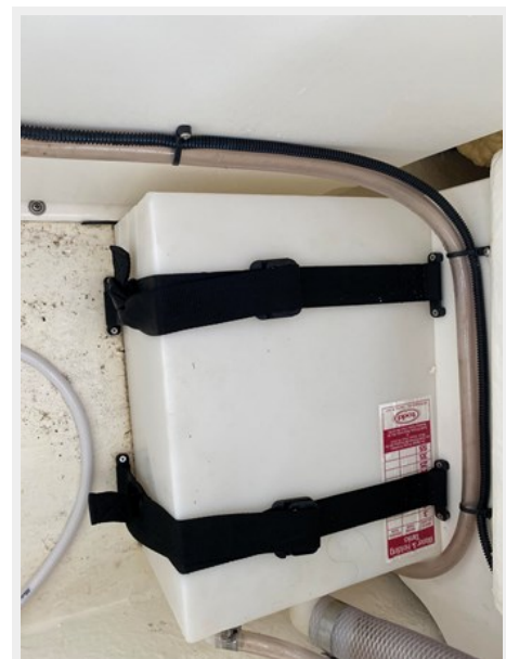
15-ADDED FRESH WATER TANK
