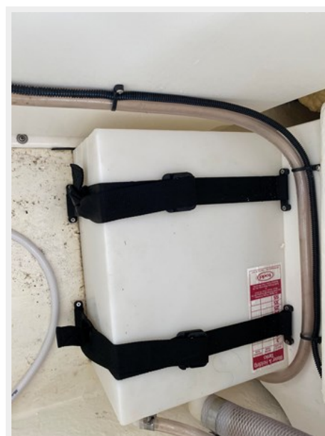
15-ADDED FRESH WATER TANK
