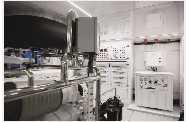
Trideck Engine Room
