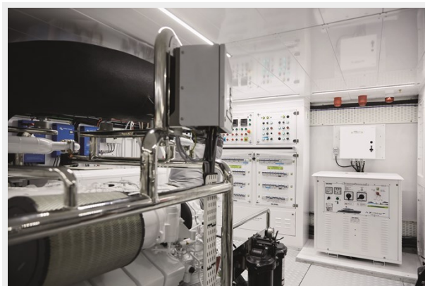
Trideck Engine Room
