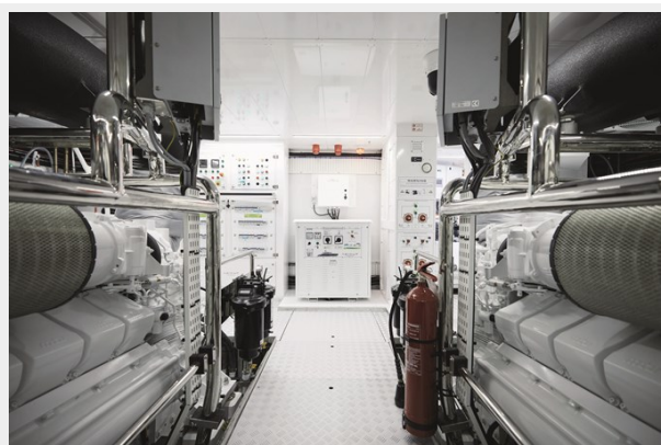
Trideck Engine Room
