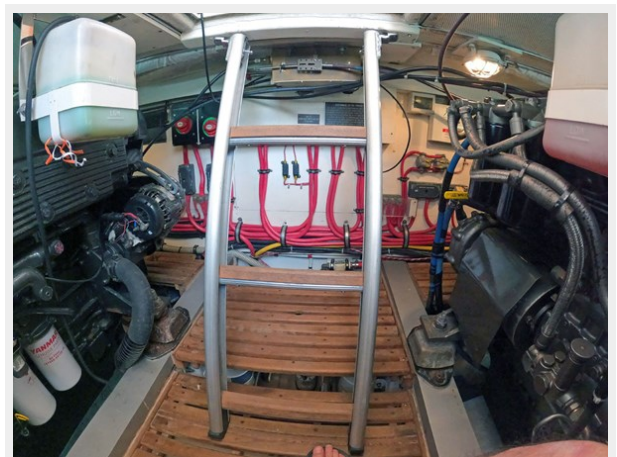
Engine Room, Fwd
