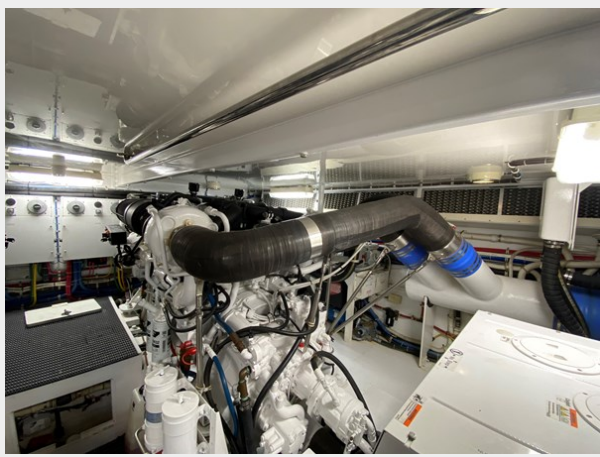
Starboard Engine Room
