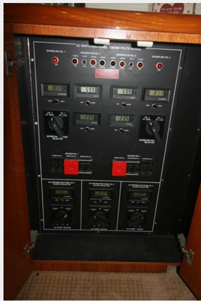
AC Switching Panel
