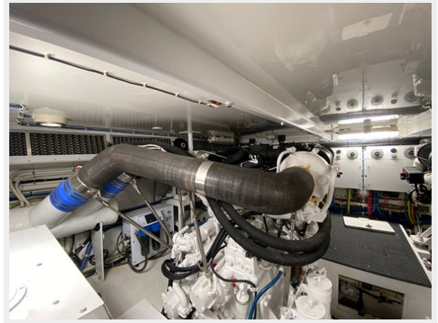
Port Engine Room
