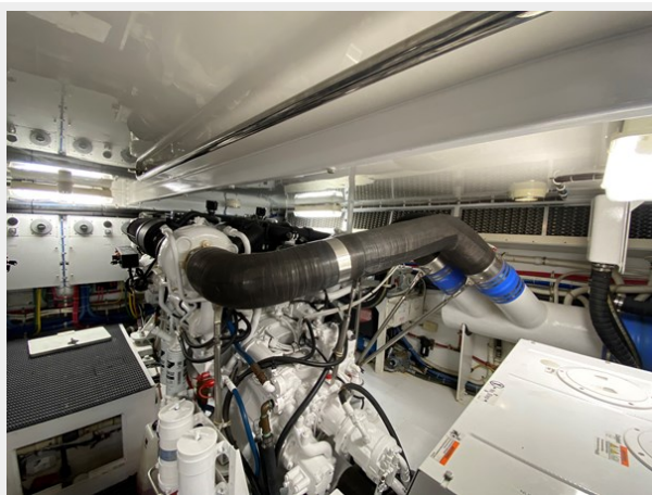
Starboard Engine Room
