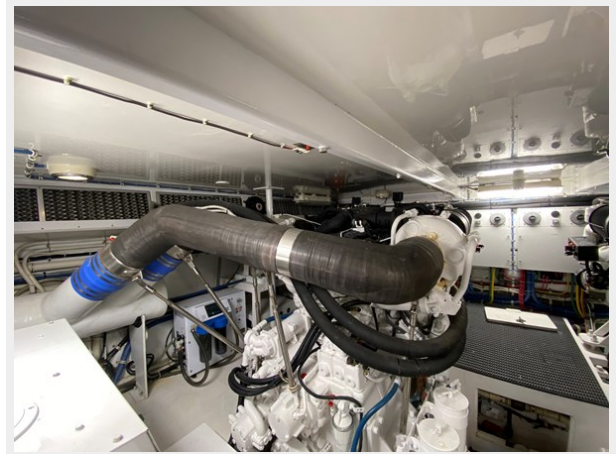
Port Engine Room
