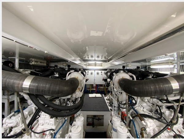
Engine Room Forward
