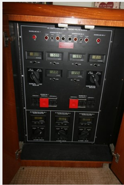
AC Switching Panel
