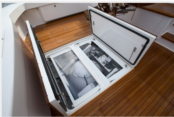
2024 72 Viking Enclosed Bridge: Seakeeper
