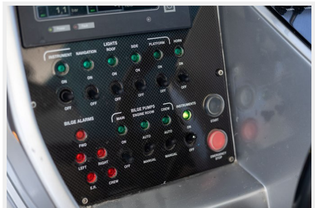
2005 PERSHING 50 - Helm Controls
