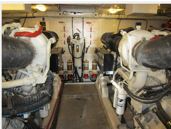
Engine Room Looking Forward
