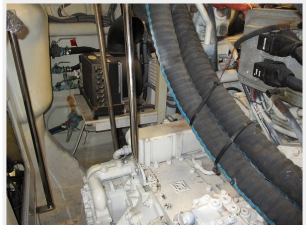
Engine Room Air Handler
