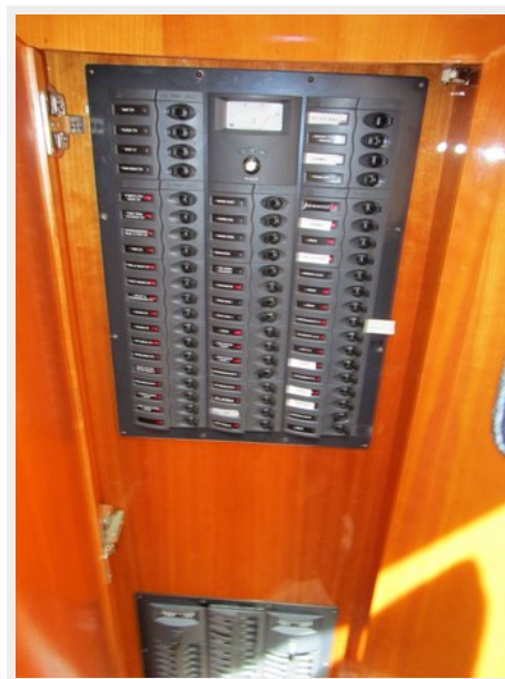
Companionway Electrical Panel
