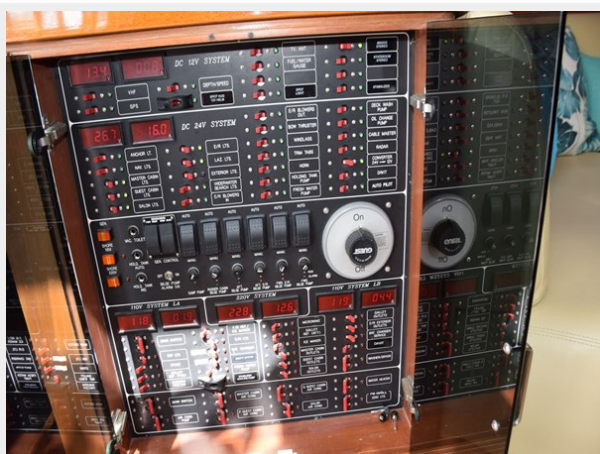
Main Switching/breaker panel
