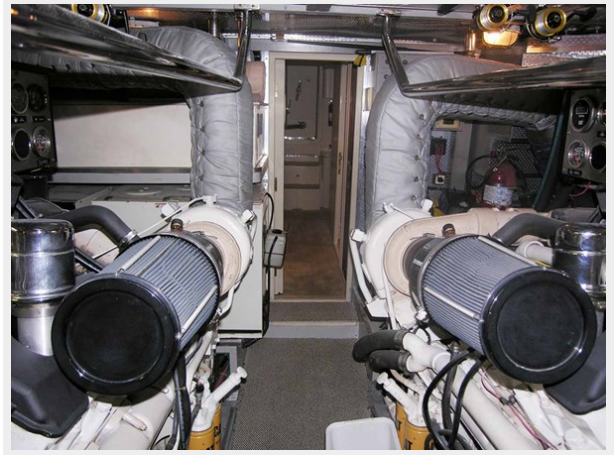
Engine Room Looking Aft
