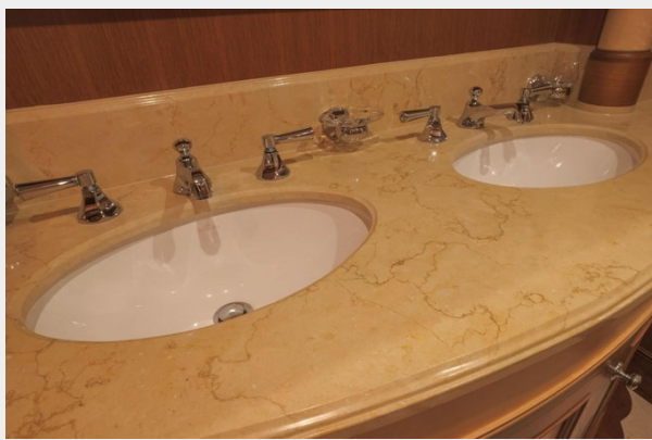
Master Twin Sinks
