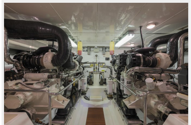
Engine Room C18's
