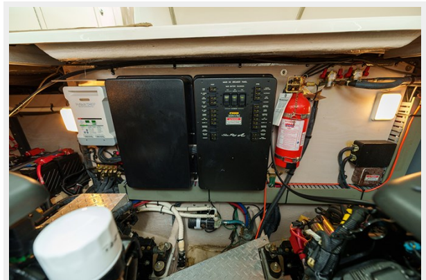
Main DC breaker panel
