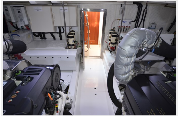
Engine Room Aft
